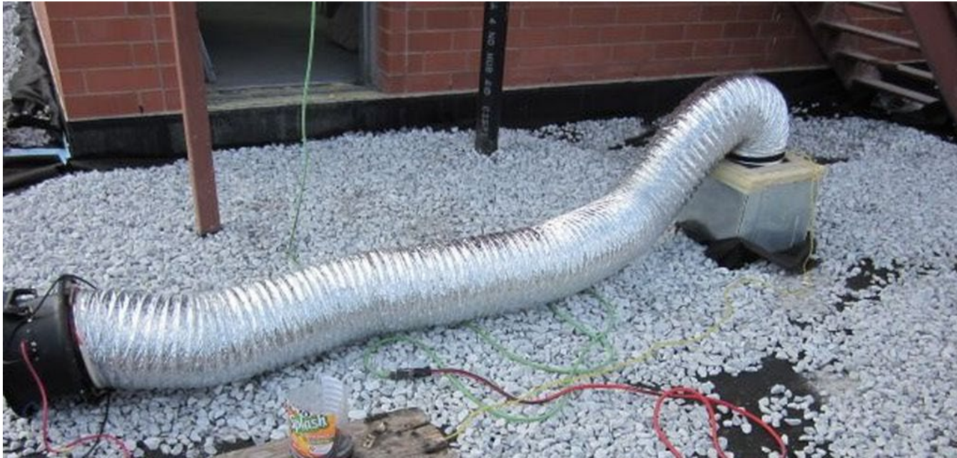
Central exhaust duct leakage test
