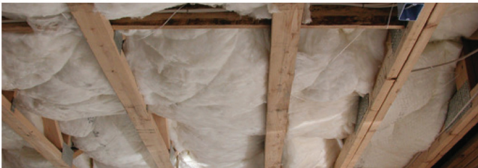
Insulation has misalignments, compression, and gaps.
